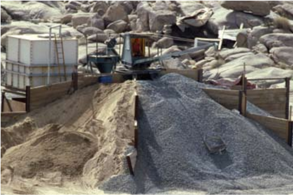
Concrete batch plant at Khamis Mushayt
