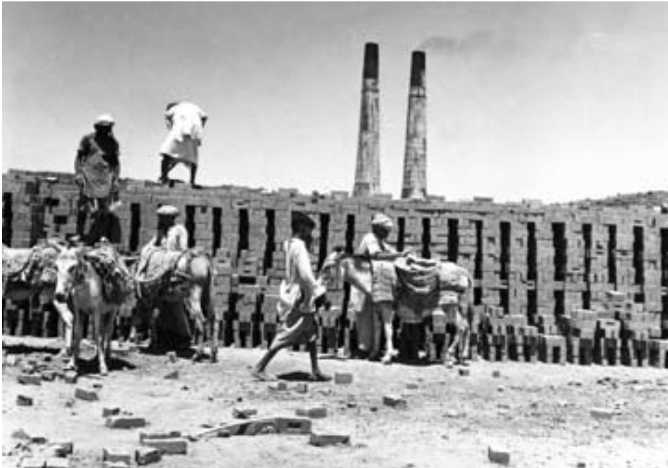
At the Kharian cantonment, workers used donkeys to move sun-dried bricks to the kilns for firing.
