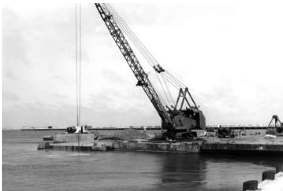
Chisimayu Port construction using a clamshell on a crane barge to remove underwater high spots, September 1966
