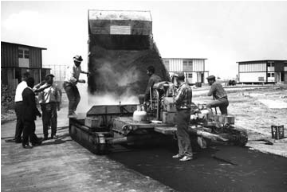
Asphalt paving during road construction in the family housing area at Karamursel, June 1970
