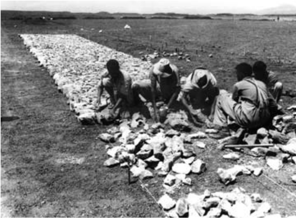
Local laborers place rocks, creating the base for the transmitter site road at Kagnew Station.
