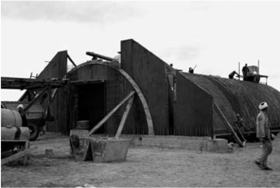
Construction of a storage igloo for ordnance at the Sidi Slimane air base, shown here in February 1957, was completed later that year.
