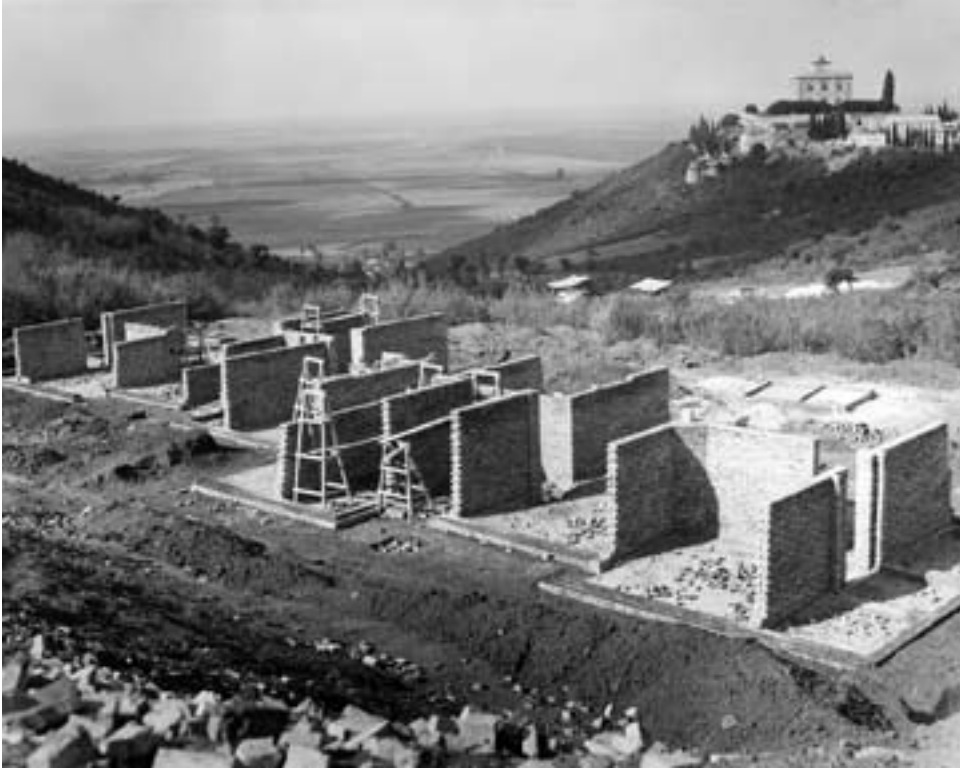
Partitions for buildings at Behshahr, Iran, were put up first while contractors waited for face bricks for the exterior walls.
