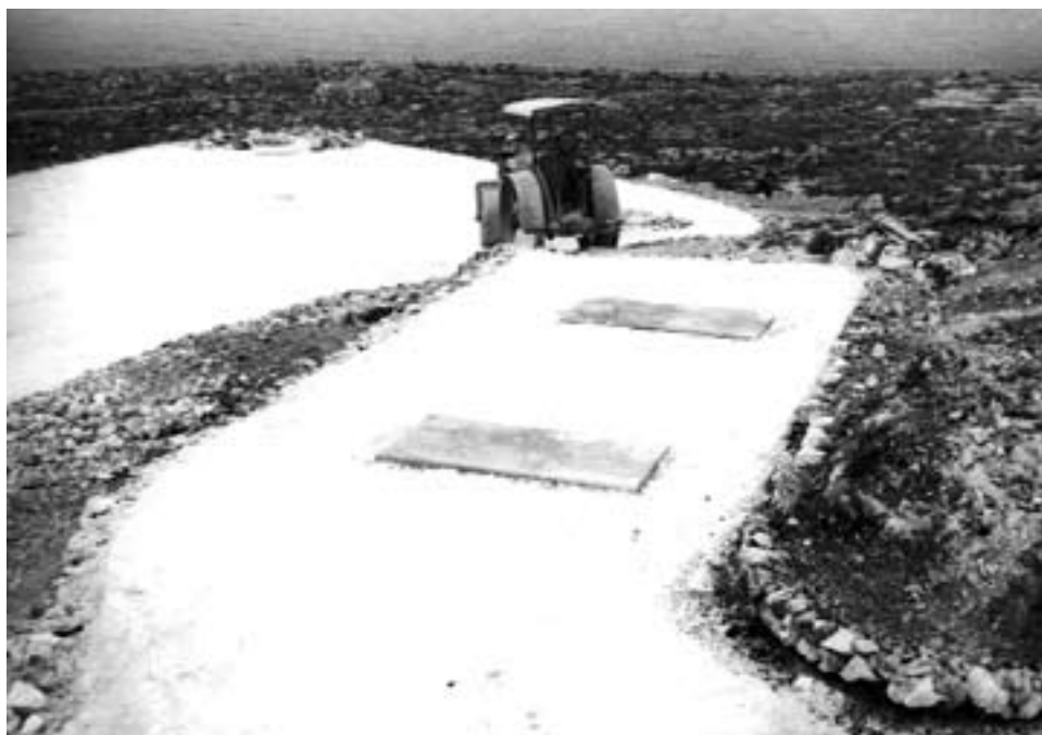
Part of the construction of the Troposcatter system on Malta, slabs upon which power equipment will be installed, May 1968
